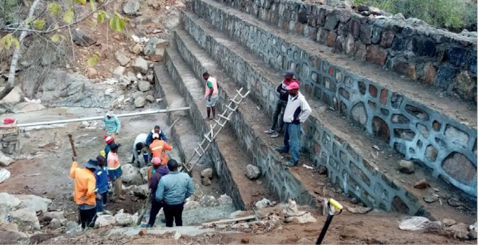
AUGUST 11, 2023: Cash for Assets workers in Ward 29 cluster 5 undertaking routine construction works at a weir dam in Zaka. The weir is now at 90% completion and the pipeline that conveys water from the weir to the garden has been fitted (centre left). © Gift Mangwende / TAKUNDA RFSA
