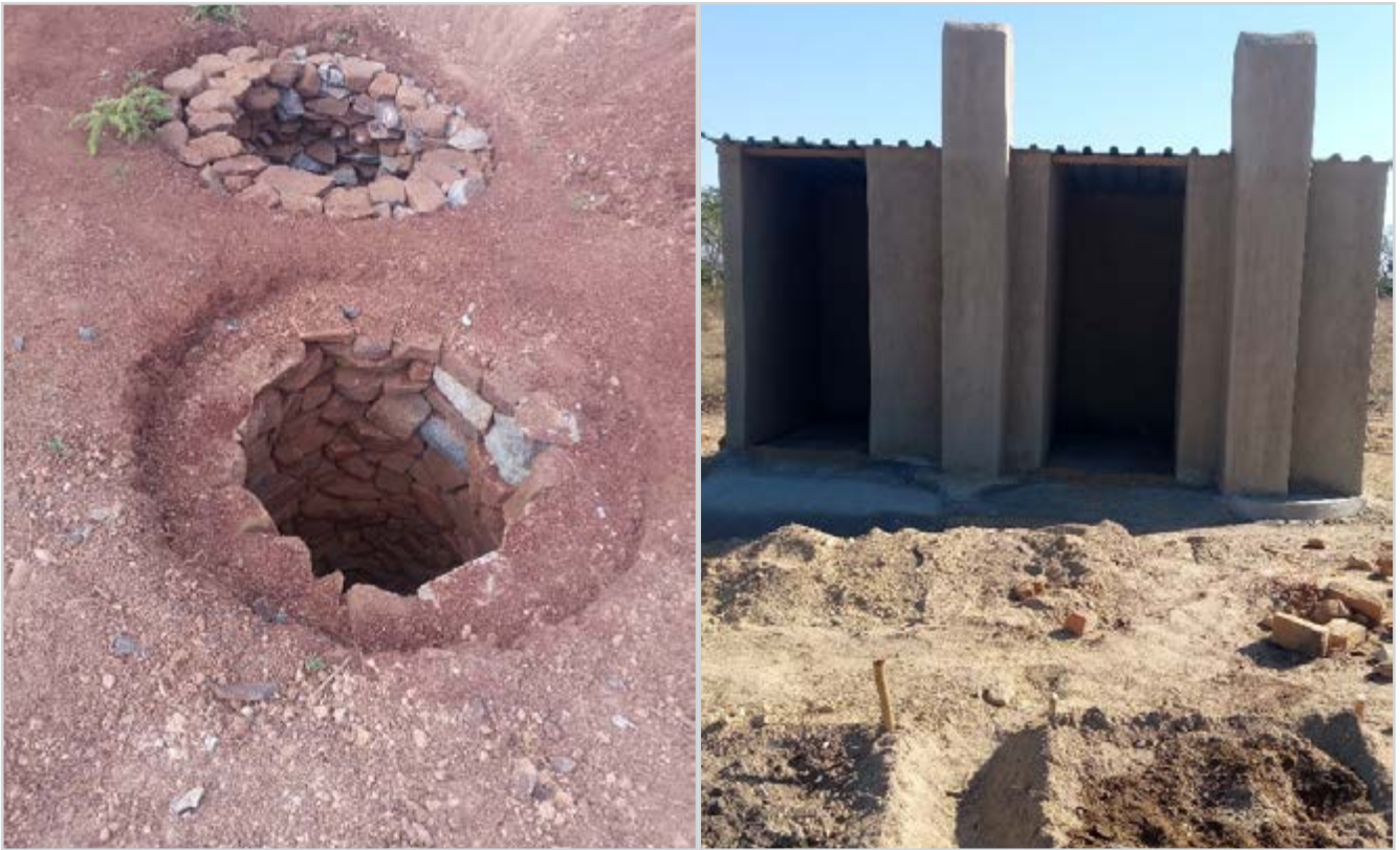
JULY 17, 2023: Members of the Ward 28 garden constructed a wheelchair friendly latrine using local resources (stones) and cement and supported by trained builders. © Jeshua Tofa/ CARE
