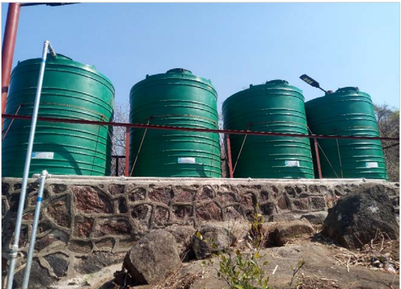
JULY 25, 2023: Newly fitted storage tanks at Dabwa piped water scheme in Ward 30 Zaka district. The system serves 5 villages, namely Muzvidziwa, Mundingi, Chavani, Nhondova and Chikwamure, Dabwa, a dip tank and Dabwa Primary School. © Jeshua Tofa/ CARE
