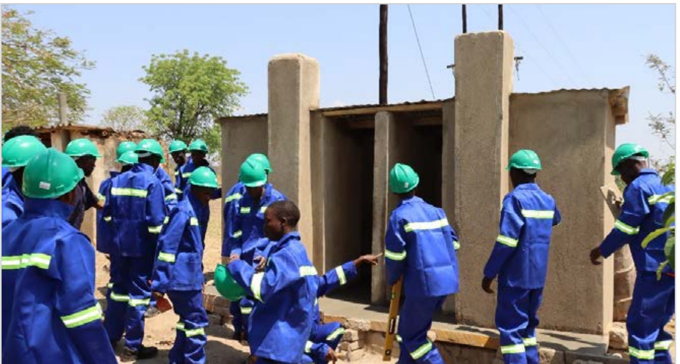
OCTOBER 17, 2022: Latrine constructed at Muzinda primary Ward 32 Zaka by Technical and Vocational Education and Training Skills Outreach participants. © Martin Chauke/ TAKUNDA RFSA
