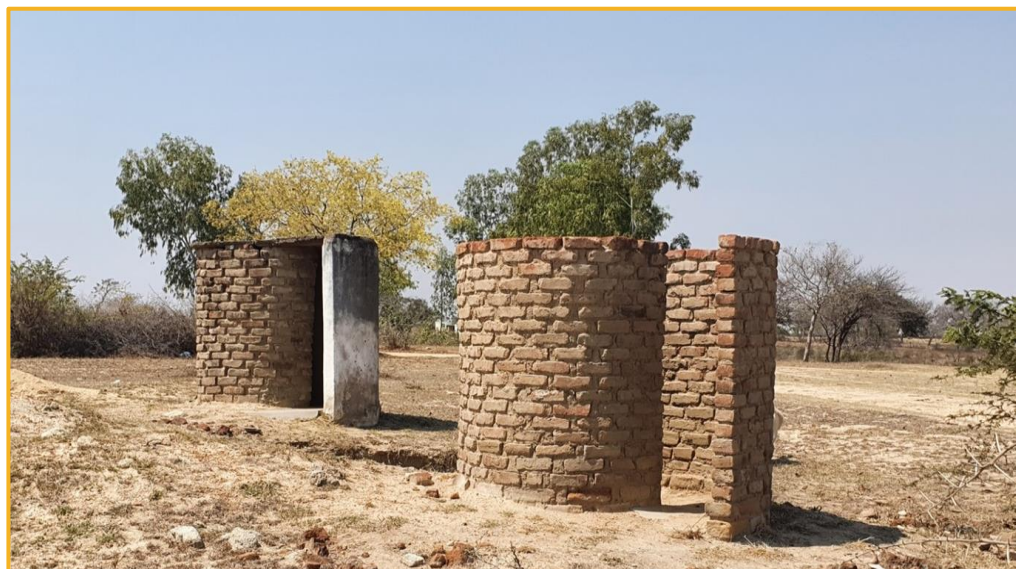
Chivi, Ward 3 Centre. The toilets at the Centre were constructed with the assistance of young people. The Youth Development Coordinator highlighted that the young men were asked to fetch water and assist with other tasks for the construction of these toilets.
