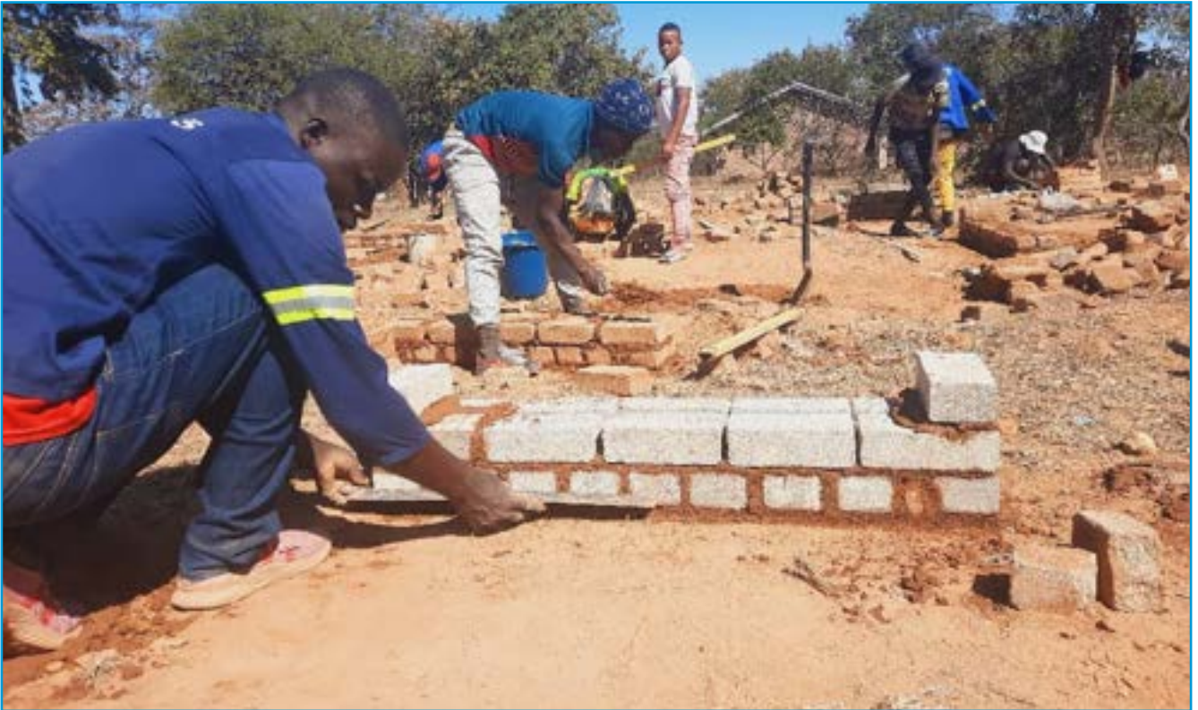
A 23-year-old BRENDON CHIMWAZA , is a brick and block laying student at Marange vocational during class practice at Marange VTC. © Nyasha Mhlanga/ CARE
