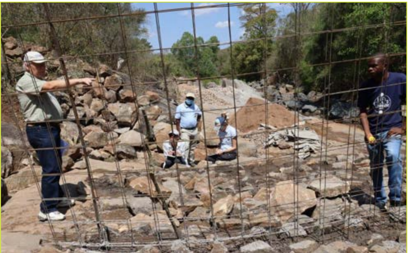
SEPTEMBER 15, 2022: USAID delegation, Darrell Smith, Nicole Van Abel, and Justin Mupeyiwa exchanging notes with the Takunda Engineer Bernard Garwi in line with the technical design of Mambwende – Tsvazvivi dam wall. © Gift Mangwende/ TAKUNDA RFSA
