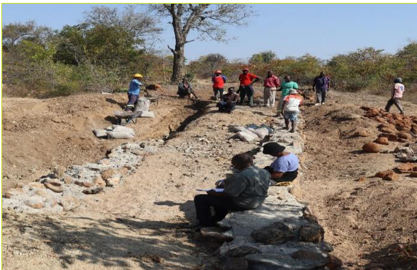
AUGUST 05, 2022: Villagers from Sengejira take a short break from building a XXX for a bridge. The bridge will connect three villages, Kwarire, Sundirai, and Dzenga, and will reduce hazards such as children drowning on their way to school. © Joshua Bhuza / TAKUNDA RFS
