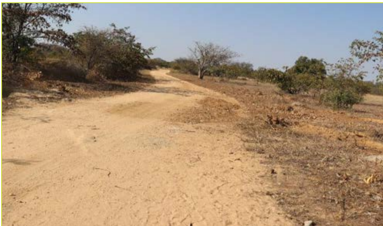
AUGUST 05, 2022: Sengejira-Ndongwe road maintenance works that included cutting and clearing vegetation on both sides of the road to ensure good visibility, cleaning of road drainage systems to reduce the accumulation of water in the road as patching of holes. © Joshua Bhuza / RFS
