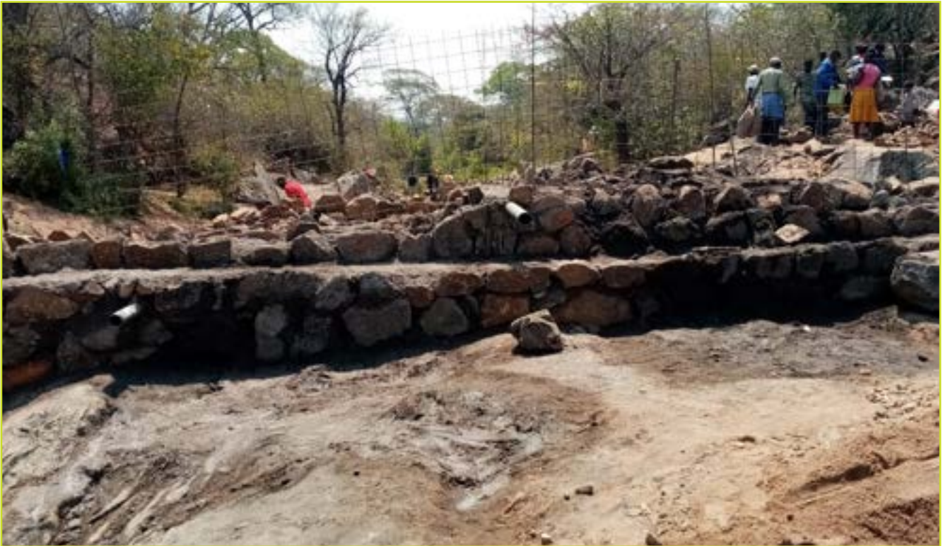
SEPTEMBER 15, 2022: A section of a newly constructed Mambwende - Tsvazvivi weir in Ward 29, Cluster 5 with two pipes installed. The bottom pipe (left) will be used to remove sediments and provide water for downstream users. The irrigation pipe (centre of photograph) will be extended and used to convey water to garden which is approximately 900m away from the weir. © Nyasha Nyamhandu/ CARE
