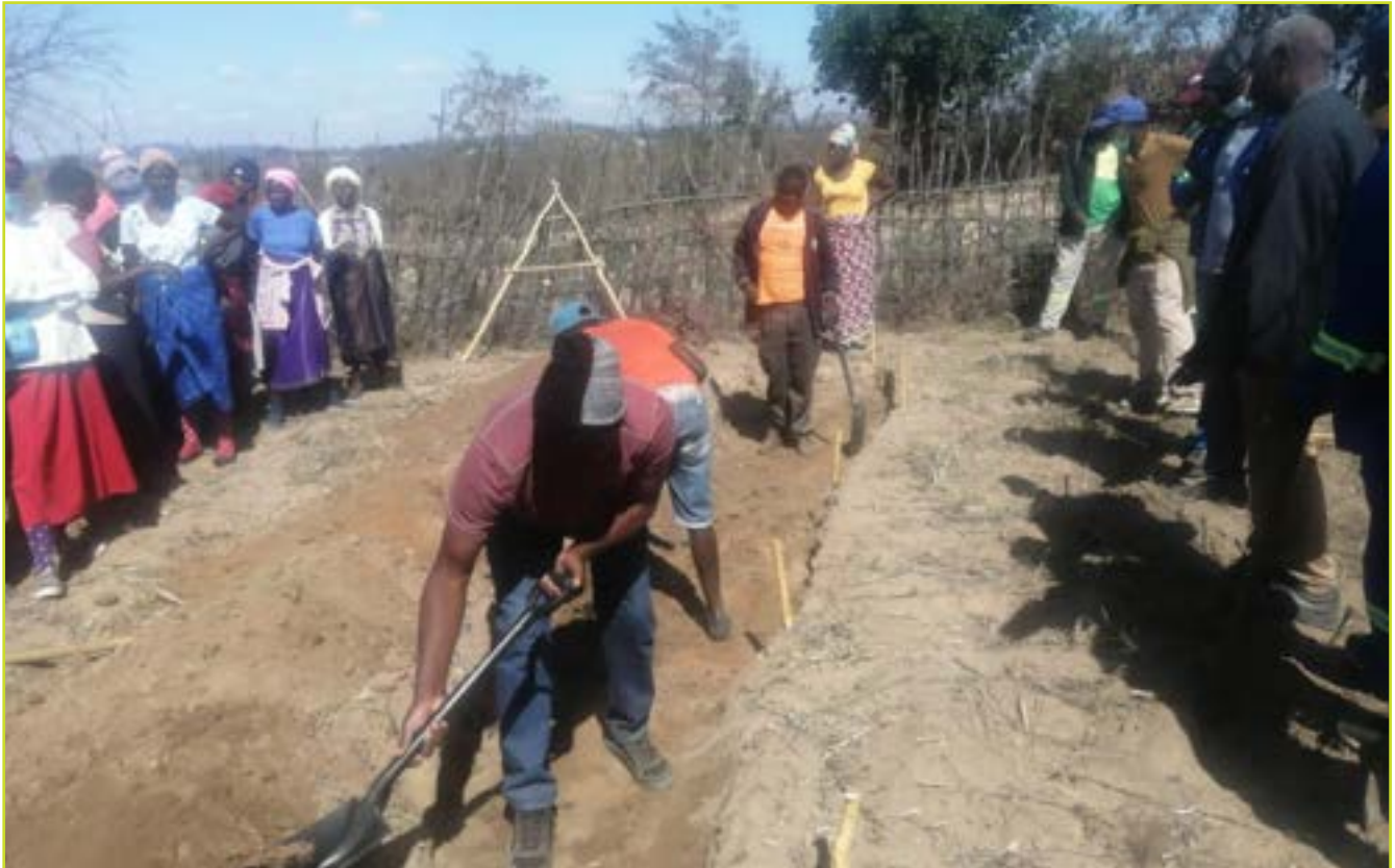
AUGUST 01, 2022: Farmers at a Farmer Field Business School shovel soil as part of a demonstration on how to construct dead-level contour. A dead-level contour structure is used to harvest water which enhances field-crop moisture retention in Ward 11 Chivi. © Polite Masara/ TAKUNDA RFSA
