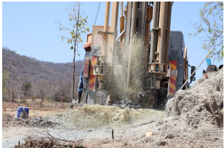
Photo 5: September 21, 2022: A high-yielding borehole is being drilled in Ward 16, Mutare District. The borehole is set to supply water for multiple uses, including domestic, irrigation/ production, and livestock watering. CARE ©2022
